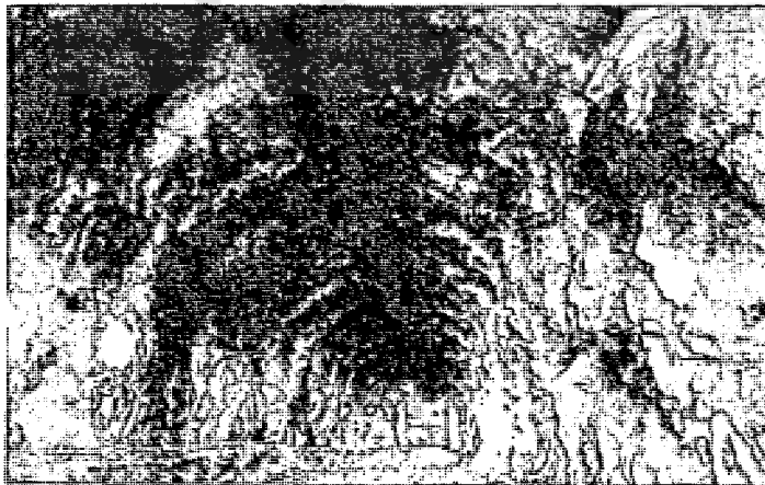
Figure 7. An example of poor blasting in a tunnel [14]
