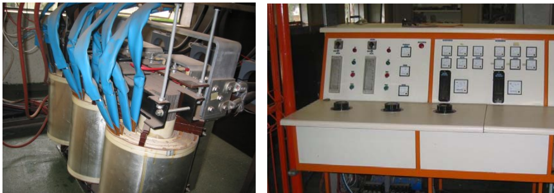
Figure 2-1: High Current Transformer (Left) and its Control Bench (Right).
