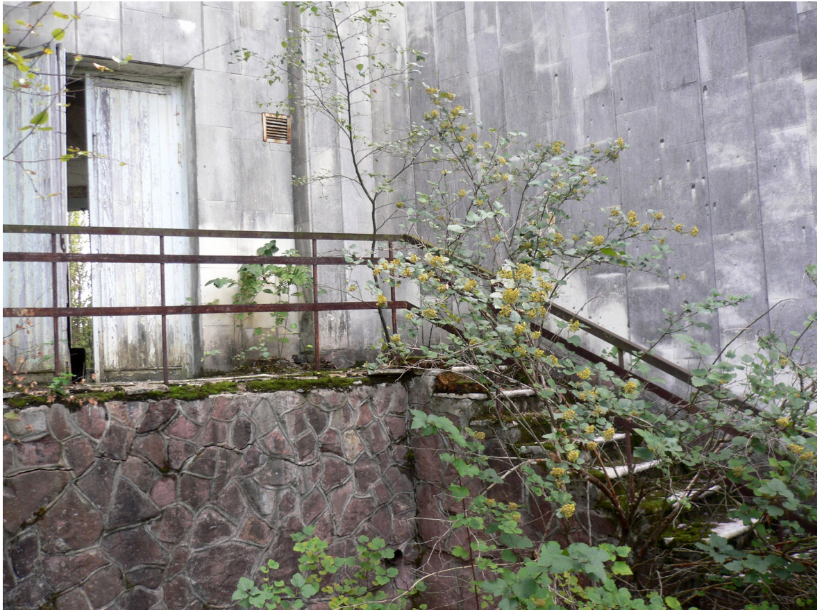
Image 64: The stairs taken from the cultural centre to the amusement park (#p1547)
