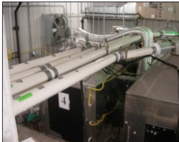
Figure B.2: Environmental Preference Chamber Ventilation System. Four 3" Inner Diameter PVC pipes carry the supply air to each of the four animal housing compartments.
