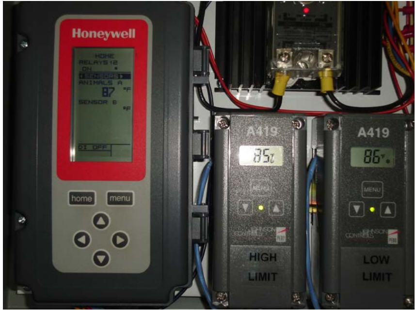
Room temperature control panel
