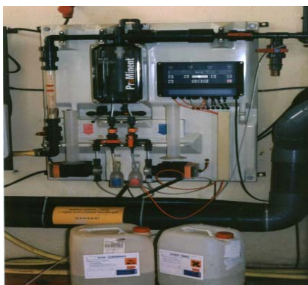
Figure 4. View of the chlorine dioxide generator.
