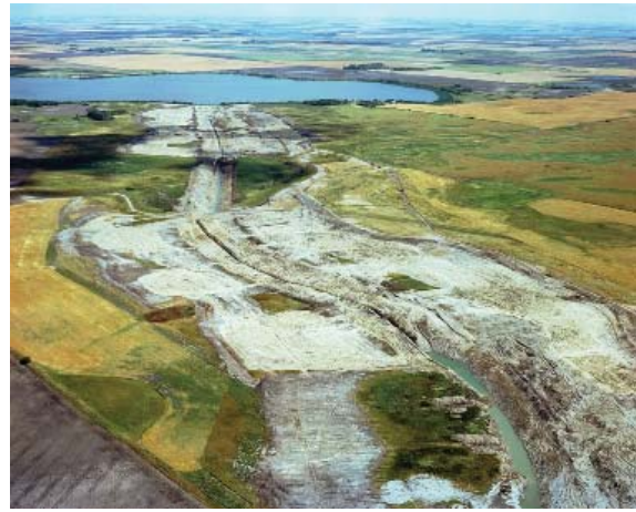
Devils Lake: A flood control diversion channel constructed by the North Dakota State Water Commission in the northeastern part of the Devils Lake watershed. (Photo by Lyle Nickly, courtesy of St. Paul District, Corps of Engineers)
