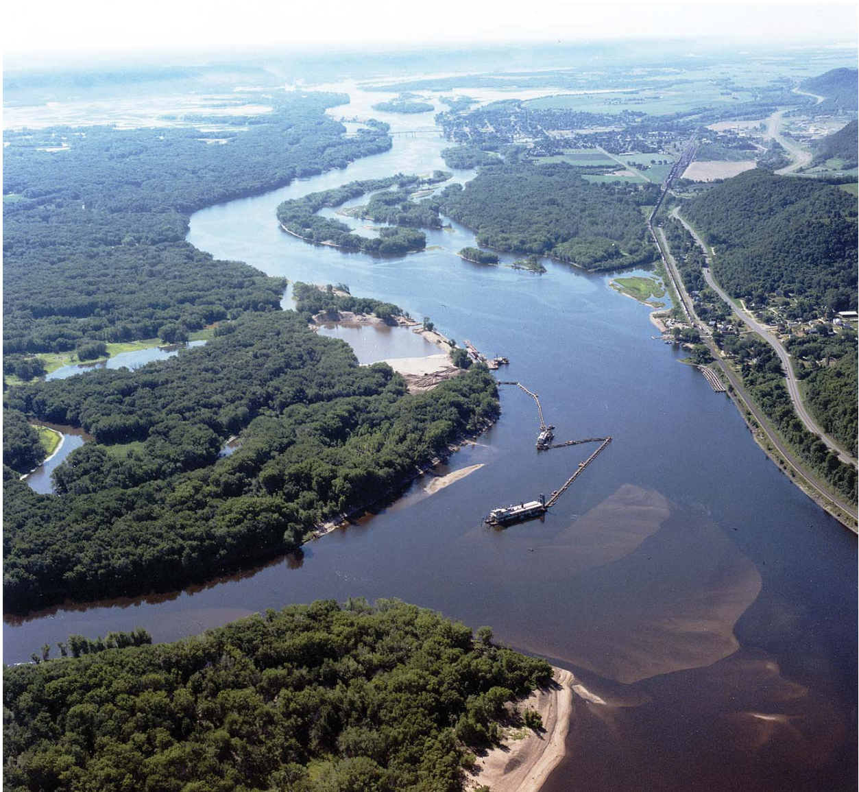
Dredging the river: A Corps' dredge in operation on the Upper Mississippi River. (Photo courtesy of St. Paul District, Corps of Engineers)
