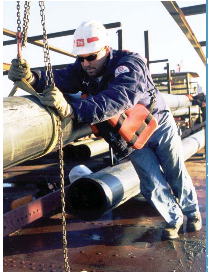
Dredging the Mississippi River: J. Skrede, a member of the crew on the Dredge Dubuque, positions pipe that will carry dredge material. (Photo courtesy of, St. Paul District, Corps of Engineers)
