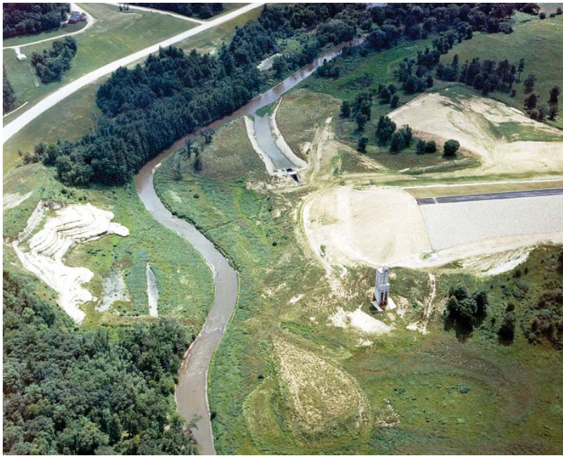
La Farge Project: The La Farge Project soon after work was suspended, 1979. The concrete intake tower is in the foreground. (Photo courtesy of St. Paul District, Corps of Engineers)
