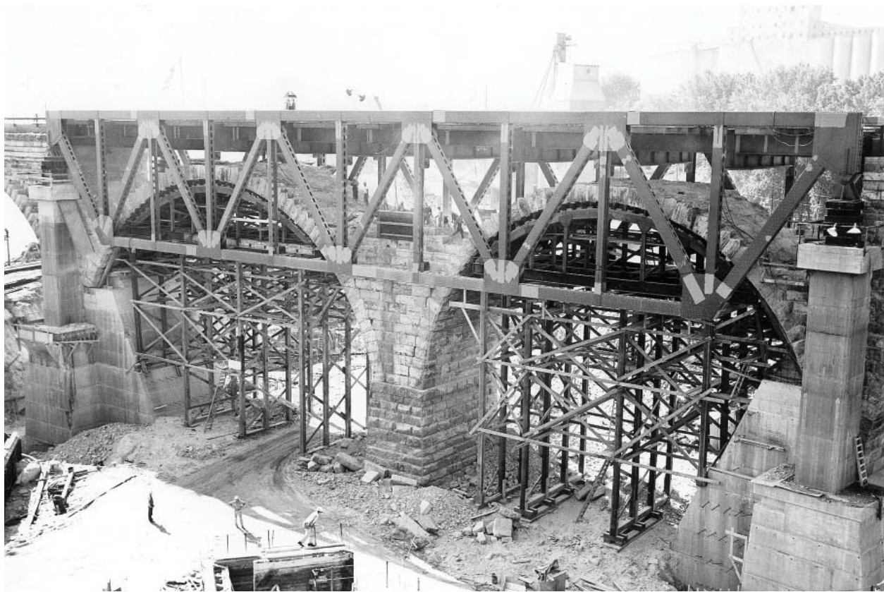
Stone Arch Bridge 1962: The Corps altering the 1880s Stone Arch Bridge in Minneapolis prior to building Upper St. Anthony Falls Lock and Dam in 1963. (Photo courtesy of St. Paul District, Corps of Engineers)
