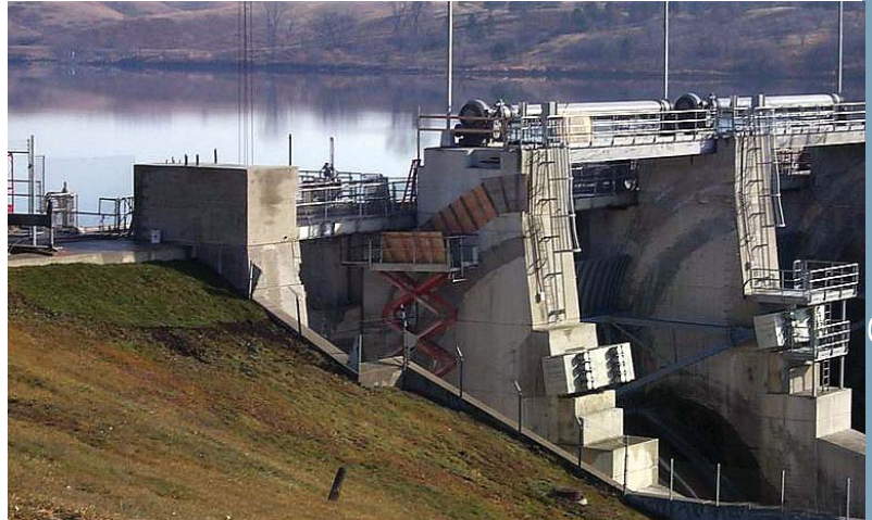
Baldhill Dam, Sheyenne River, N.D.: The district operates and maintains approximately sixteen multi-purpose reservoirs, mainly for flood control, and another thirteen locks and dams for navigation. (Photo by Ken Horner, courtesy of St. Paul District, Corps of Engineers)
