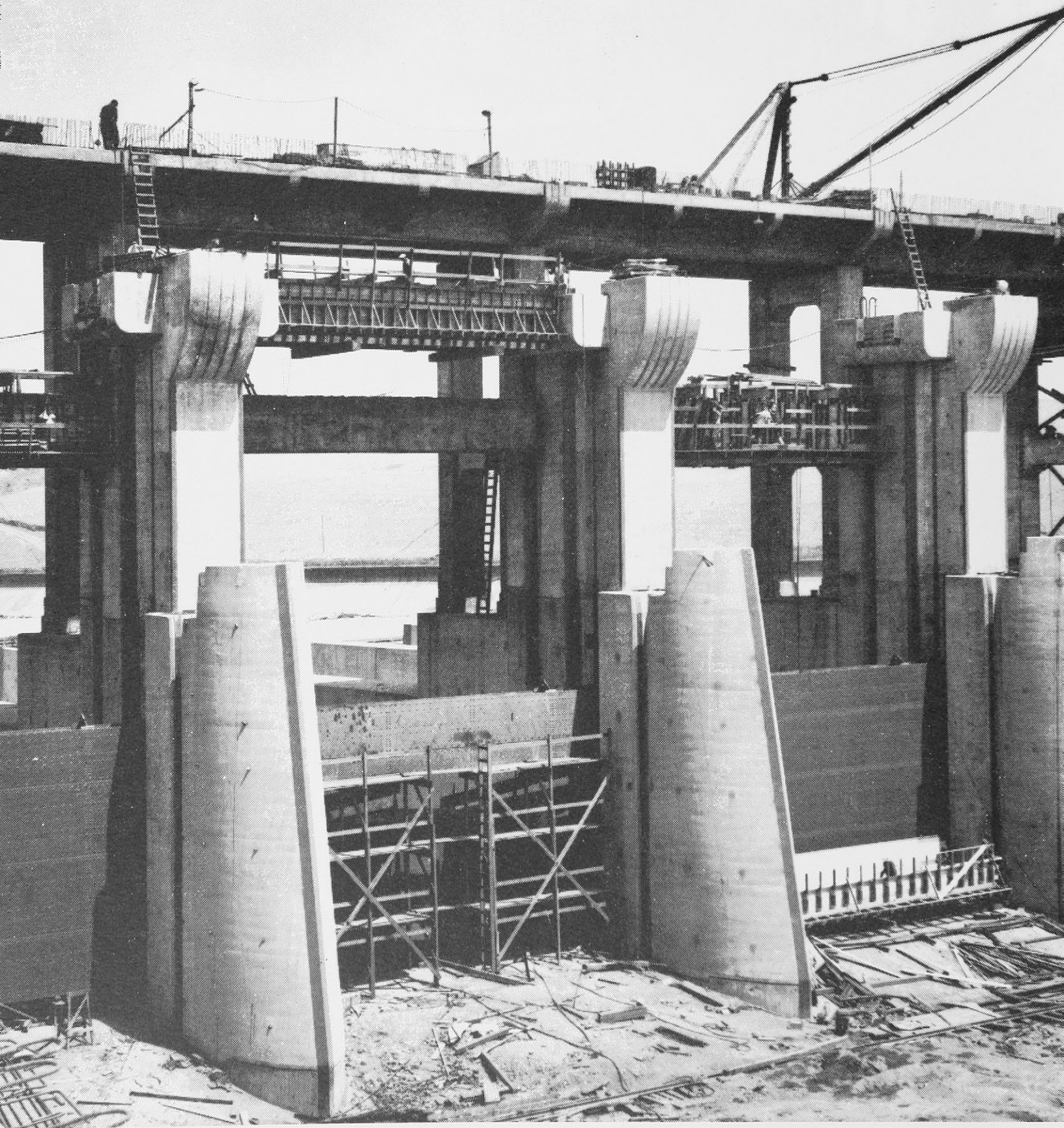
This is how the spillway looked in 1937; at right, the cover of the first Life magazine.
