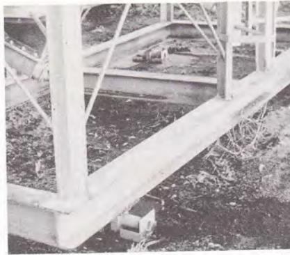
Load cells under feed bin.
