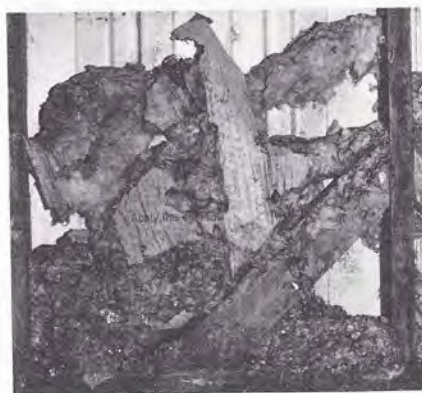
Figure 1. House mouse damage to fibreglass bat insulation inside a wall of a swine finishing building.
