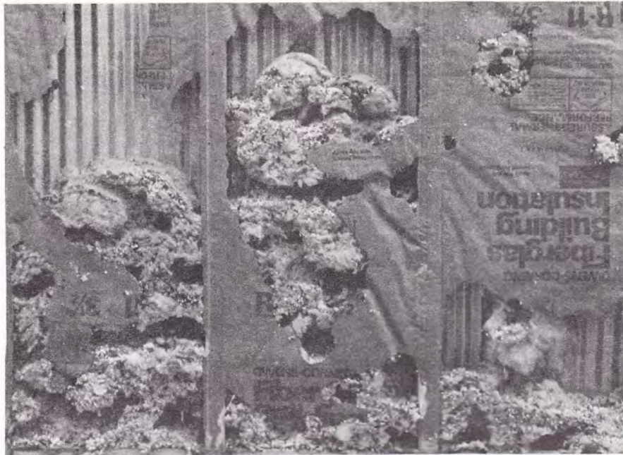
Figure 1. House mice damaged the insulation in this wall panel in a laboratory experiment at the University of Nebraska-Lincoln. The damage occurred in 6 months.
