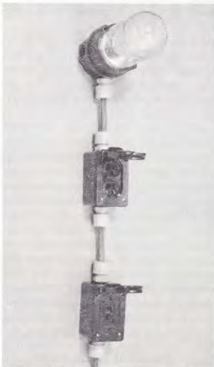
Figure 1. UF cable entering dust- and water-tight, nonmetallic boxes in corrosive environments must be secured to structure within 8 inches of box.
