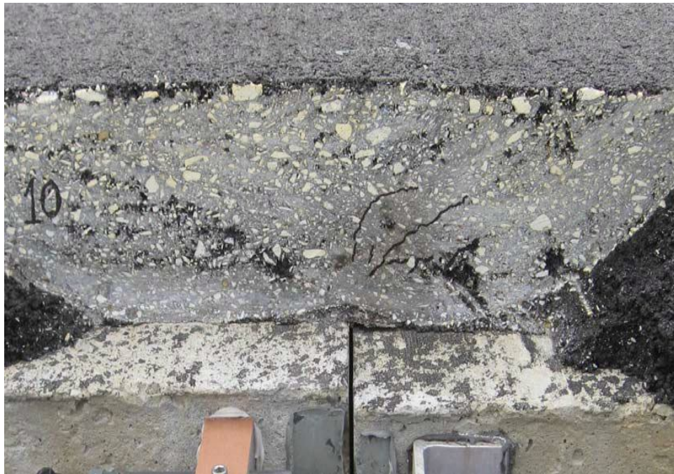
Figure 2-3. Asphalt Concrete Cracking (Braham, 2008)
