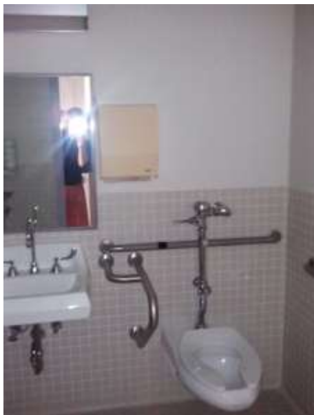
Figure 5-Shared toilet in older room provides the only place for staff and patient(s) to wash hands.
