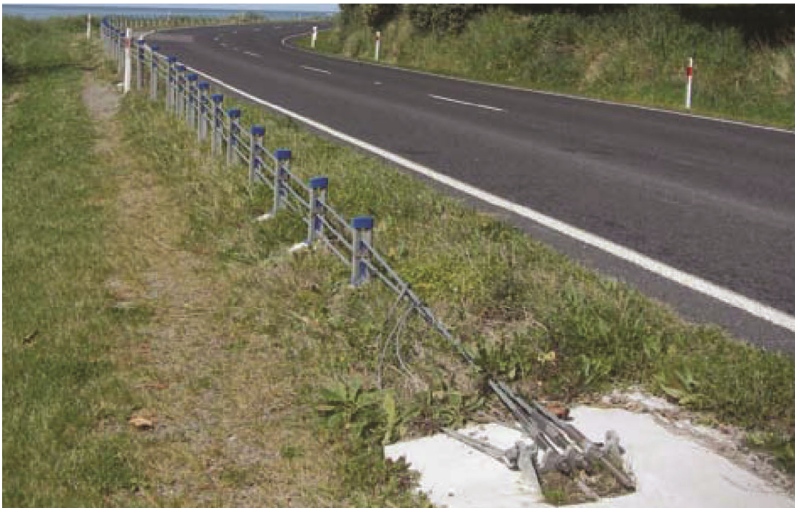
Figure 7. Safence End Terminal
