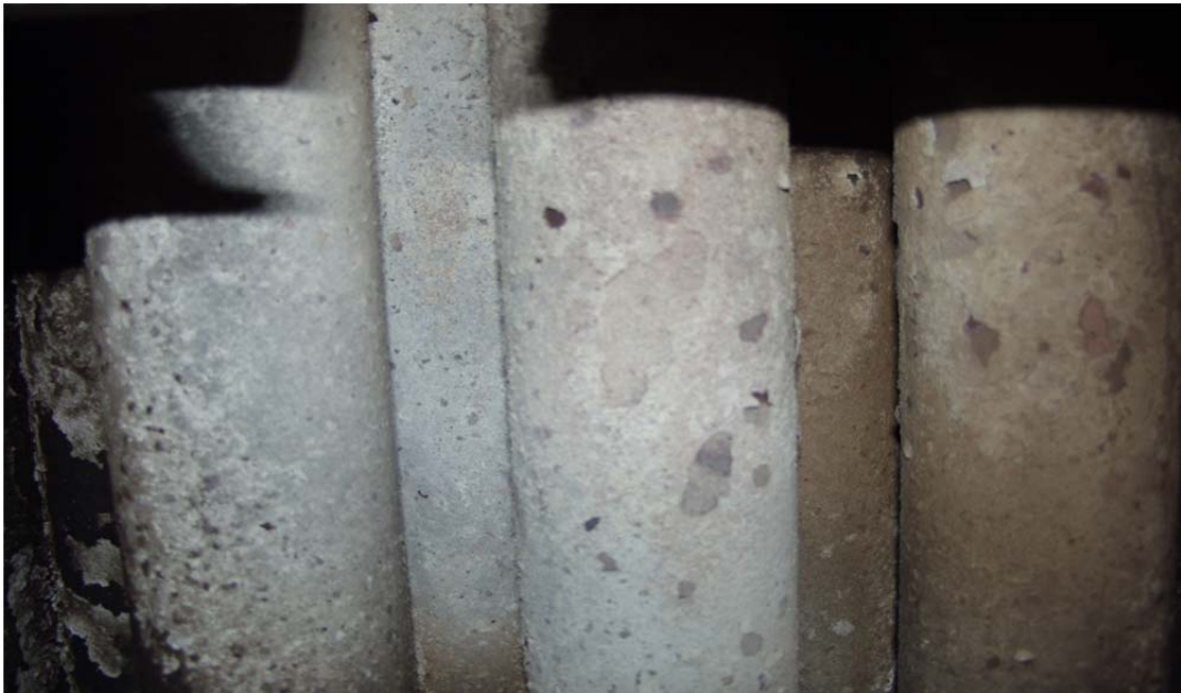
Figure 3.7. Fouling of Heat Exchanger Pipes.
