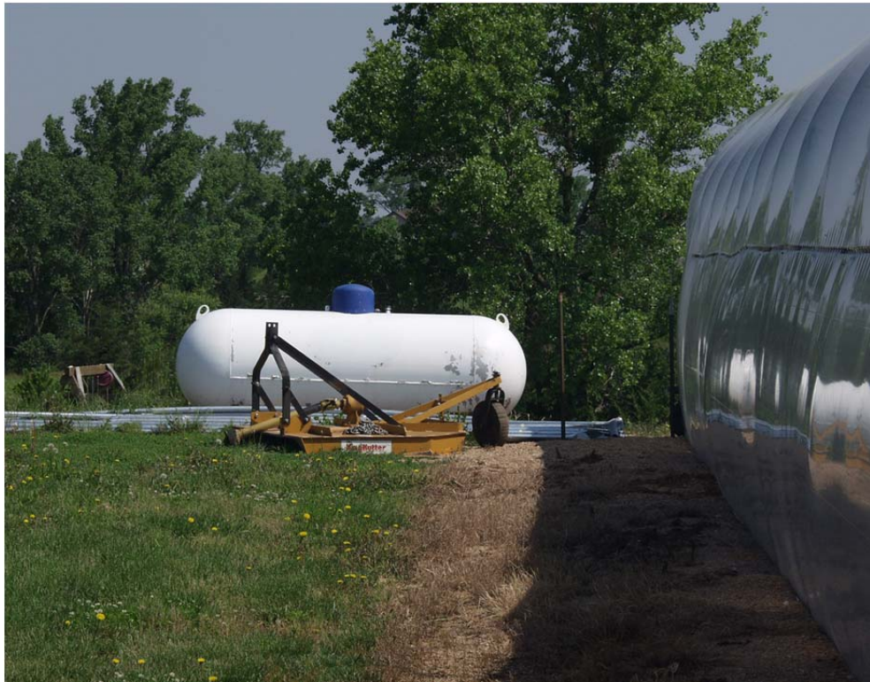
Figure 1.7. Propane Tank for supplying fuel to the Greenhouse.
