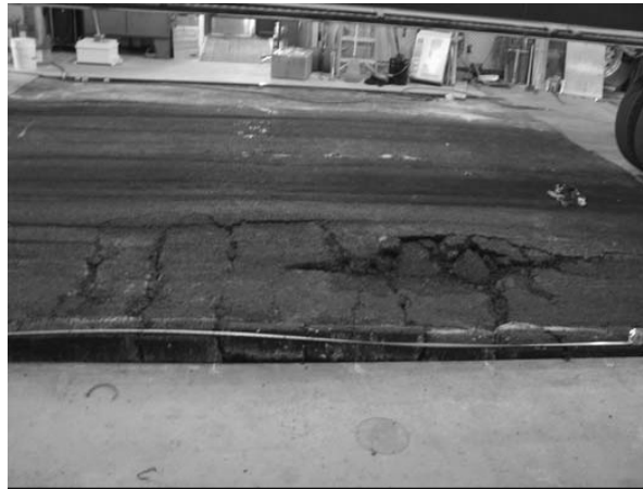
Figure 2.12 - Weak asphalt section built with uncrushed gravel (White et al., 2006)
