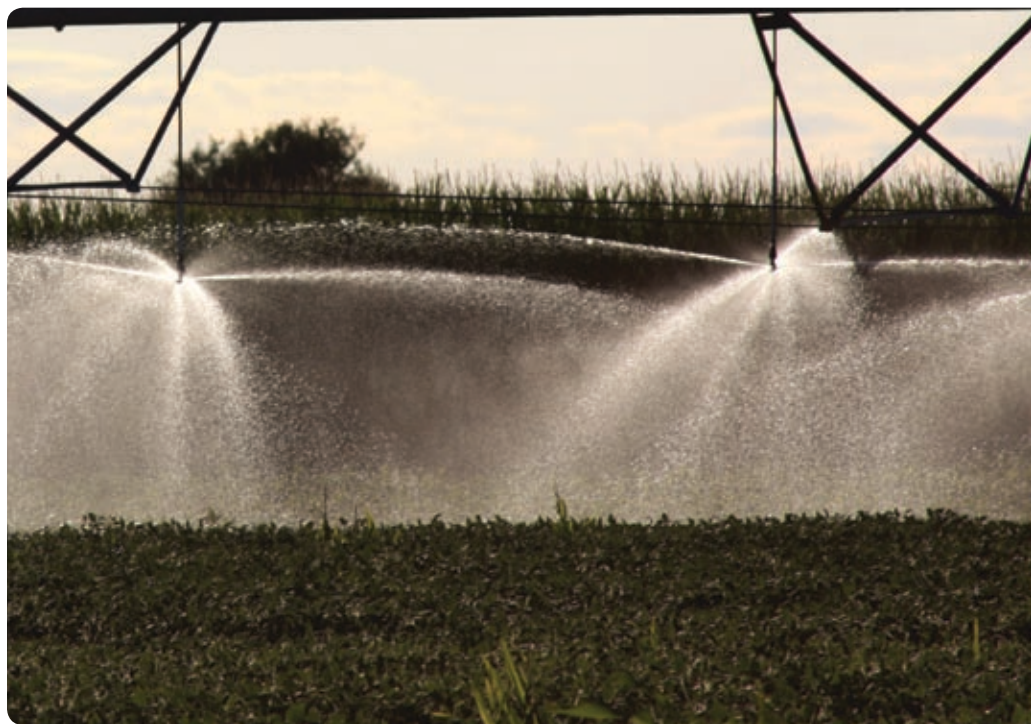
Center pivot with low-pressure spray nozzles and hose drops
