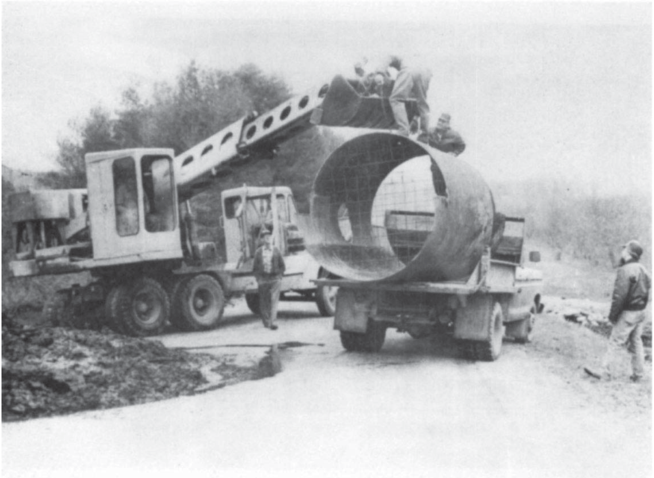
Figure 3. A 6 ft. diameter large culvert with extended ends used in fencing back unstable substrate.
