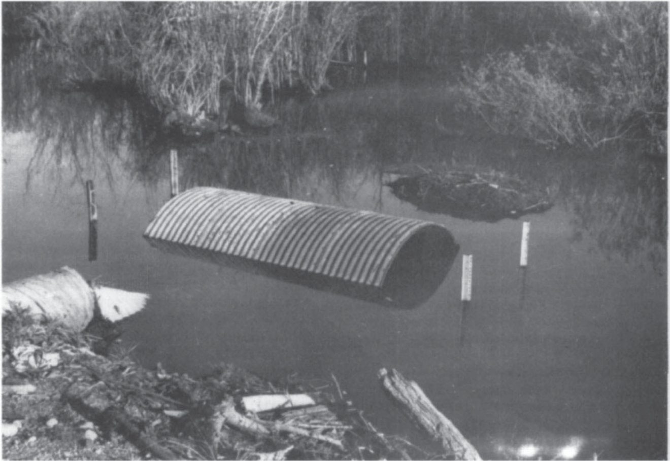
Figure 6. T-culvert shown in Figure 3 in place. Metal posts support plywood fencing against the extended culvert ends.
