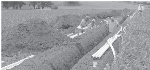
Subsurface drip irrigation being installed at the West Central Research and Extension Center.
