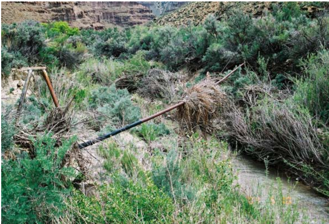
Figure 3. Although this pipeline crossed above the bankfull channel indicators, it was not high enough to escape more extreme floods.
