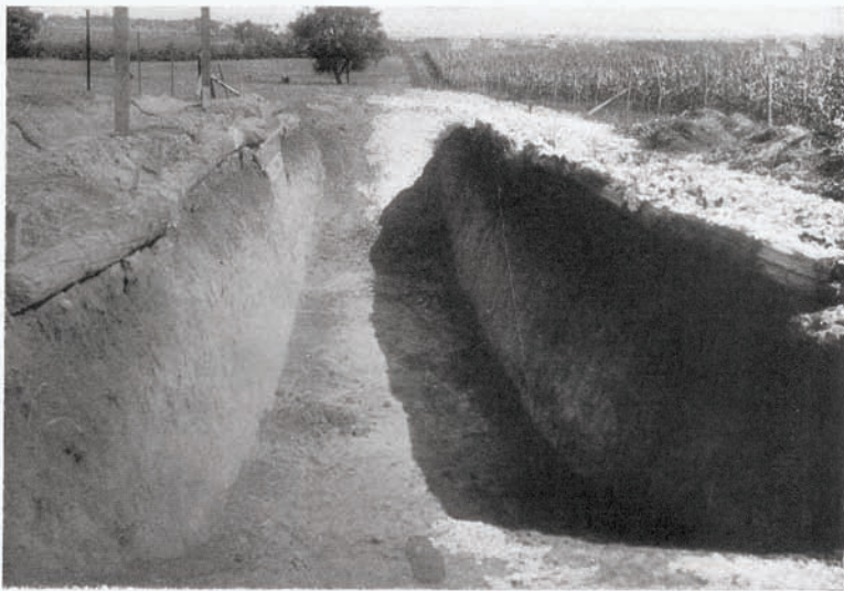
FIG. 26.—A trench silo ready for filling. This makes a very practical and inexpensive silo.
