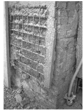
Figure 4 Failure of jacketing
