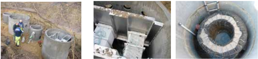
Figure 1. From left to right: installation of drainage filter system; lamella cassettes; basket with shell sand filter matrix.
