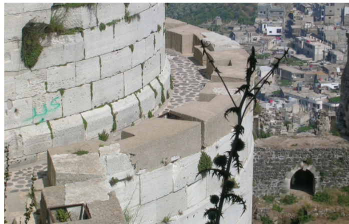
FIGURE 3-42: GRAFFITI ON THE WALLS OF THE WORLD HERITAGE SITE CRAK DES CHEVALIER 46
