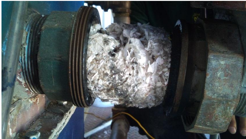
Figure 21. Shredded MSW clogging
