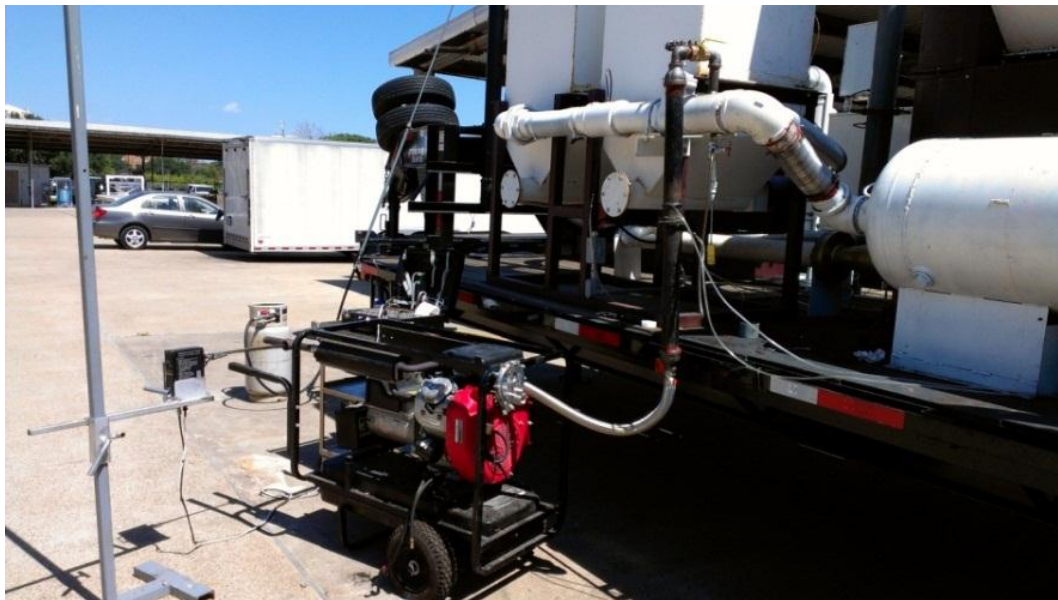
Figure 26. Gasification system connected to a 10 kW generator
