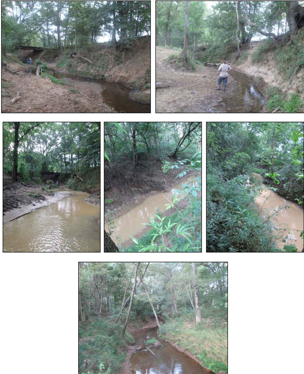
Photogroup 4-41 West 4 depicting general stream characteristics and water surface appearance. All individuals featured are SFASU and CES staff. Top left: 30-m transect, upstream, August 2012; Top right: 30-m transect, downstream, August 2012; Middle left: 30-m transect, upstream, July 2012; Middle center: 150-m transect, downstream, July 2012; Middle right: 300-m transect, upstream, July 2012; Bottom: 150-m transect, downstream, August 2012.
