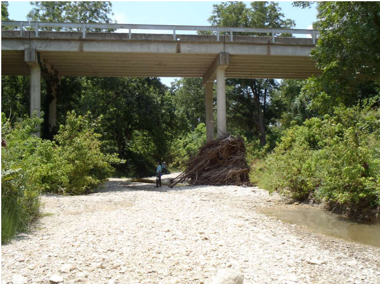
No flow condition (ponded) in Reese Creek, Bell County.
