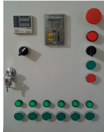
Fig. 13. Front view of the control panel. Source: Authors
