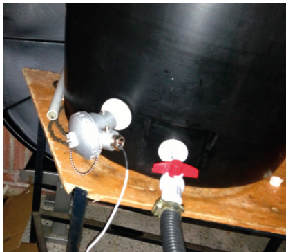
Fig. 2. Installed temperature sensor. Source: Authors
