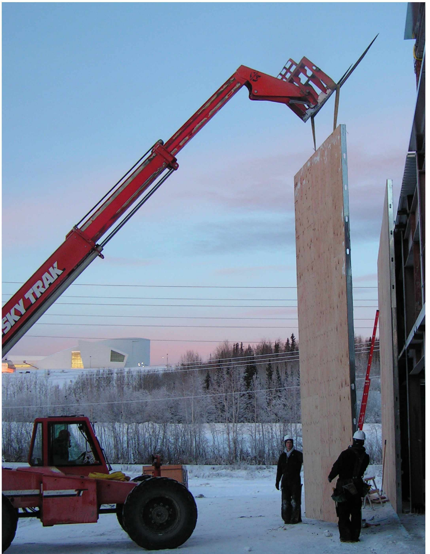
The CCHRC research and testing facility under construction. Photo credit CCHRC archives.
