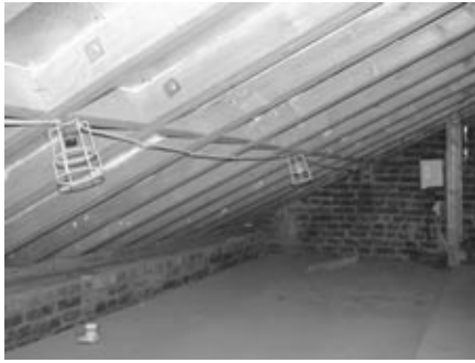
Fig. 3. Air infiltration was reduced at the LEVH through a complete rebuild of the roof; silicon sealant was used at the joints between insulation panels and roof joists.
