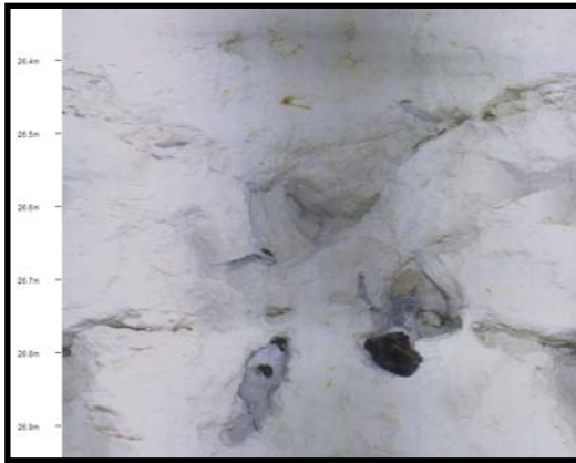
(a) Multiple fractures at 83.7 to 84 m AOD
