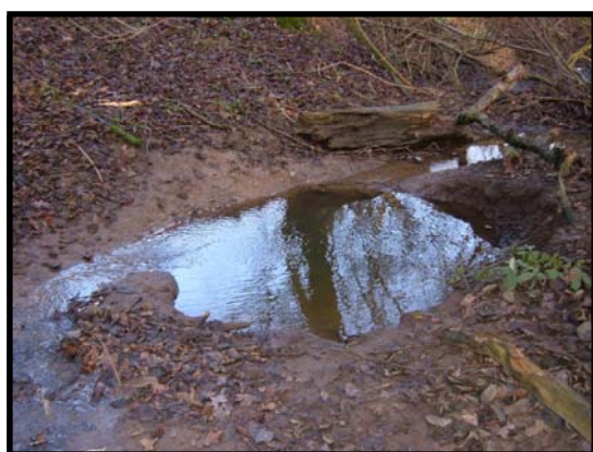
Figure 4.4: Ponding at a sink point
