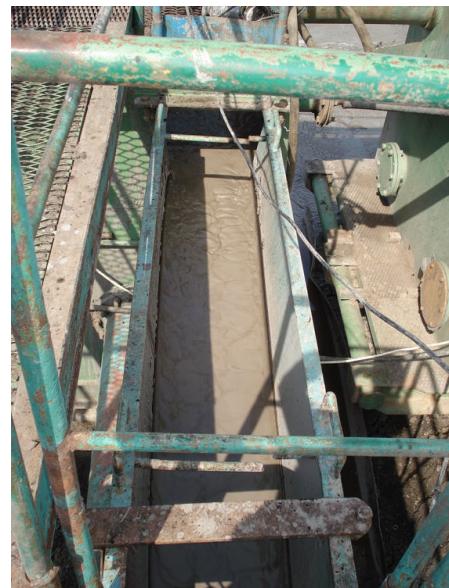
Figure 1. Unsealed channels of a pumping-circulatory system
