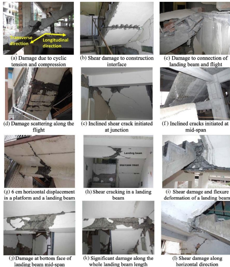
Figure 3. Common earthquake induced staircase damages
