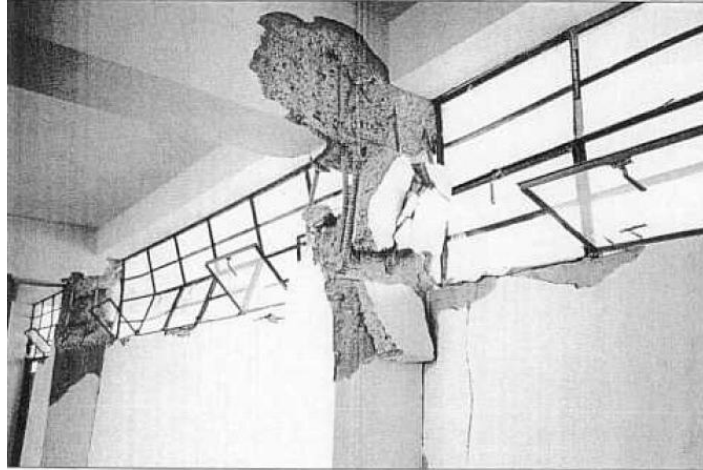
Figure 1. Short column failure
