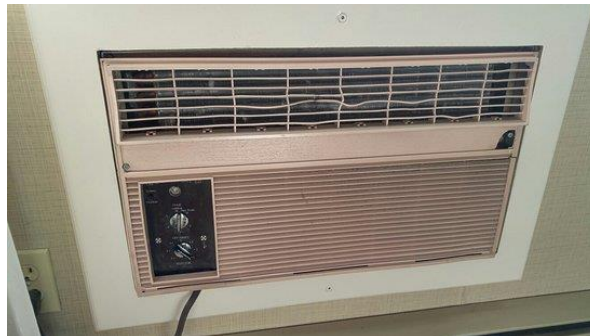
Figure 6. Old air conditioning unit
