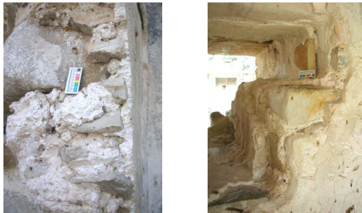
Fig 7.5. Thick pure lime plasters used as joining mortars and renders. Left: original wall at Temple of the Foliated Cross (cross section of collapsed wall). Right: original wall in House D of the Palace.
