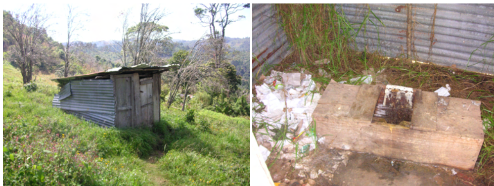
Figure 22 The worst of latrine construction and maintenance in El Mash (school house latrine)
