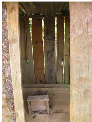
Figure 21 The best of latrine construction and maintenance in El Mash (private latrine)
