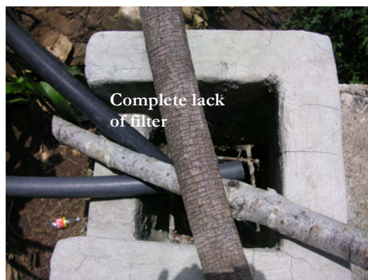
Plate 6 Elements of a poorly constructed rainwater tank (images of tanks constructed during a government-led project in El Mash)
