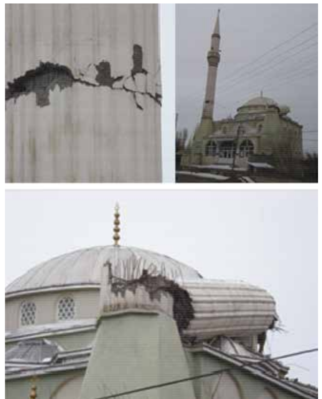
Figure 23. Local damage and two totally collapsed minarets of a mosque in Erciş
