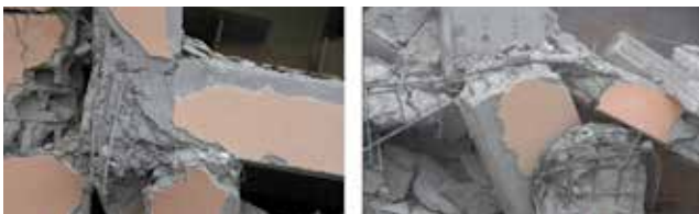
Figure 11. Typical failure at the joints of a multistorey building in Erciş
