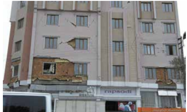
Figure 17. Diagonal damage patterns occurred at the infill sandwich walls in city of Van
