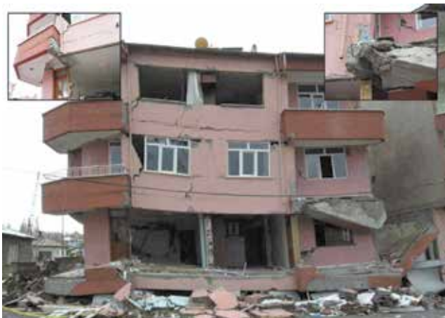
Figure 16. Damage due to selection of an improper structural system in Erciř
