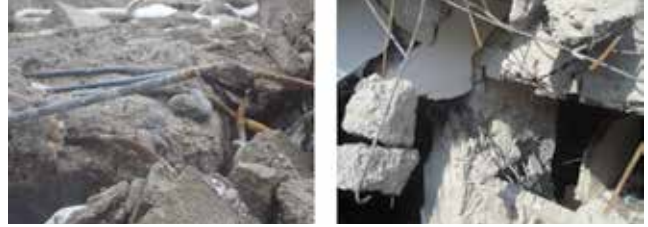
Figure 27. The use of plain reinforcement as longitudinal rebars in RC beams and columns
