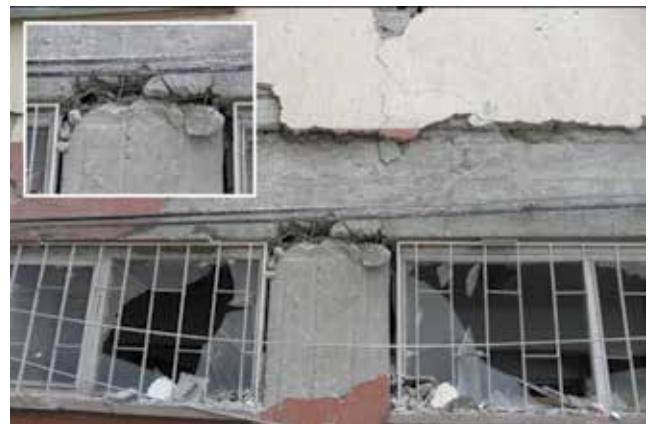
Figure 13. Shear failure at the top of the column due to short shear span in Van
