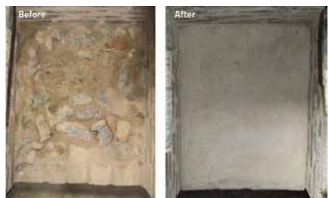
Figure 9. Appearance of the floor area before and after conservation treatment [4]
