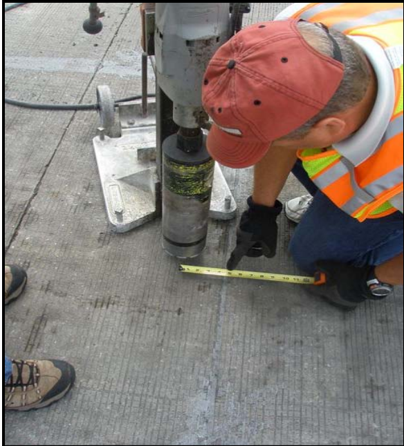
A – Sensys representative indicates the location where sensors should be installed (about 5 inches from the leading edge of loop).
