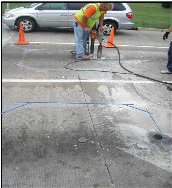
C – General view of the three lanes. An off-centered sensor was already installed in the near lane, and one more is being installed in the far lane.
