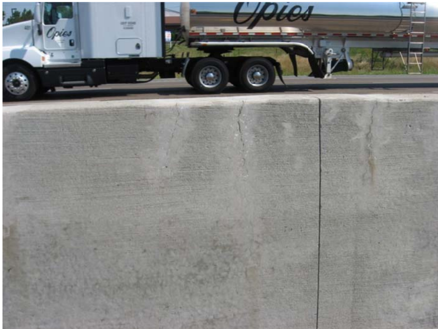
Figure 18. Cracking in the barrier wall could be quite frequent, occurred regardless of contraction joints, and initiated at the top of the barrier wall.
