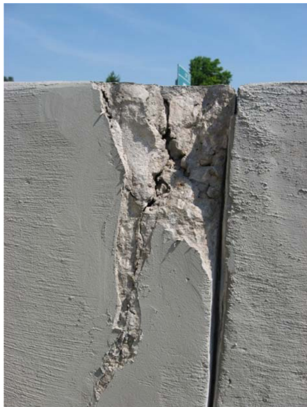
Figure 19. A severe crack in the barrier wall. Poor consolidation can be seen in the cracked off portion, and the contraction joint is not cracked through.
