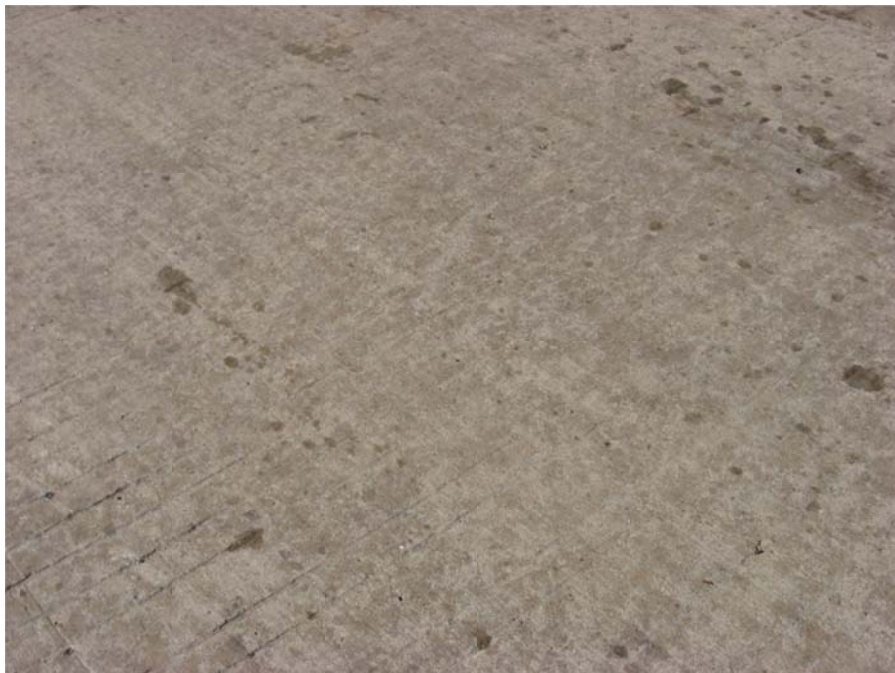
Figure 12. Crazing and poor tining on exit ramp jointed concrete pavement.
