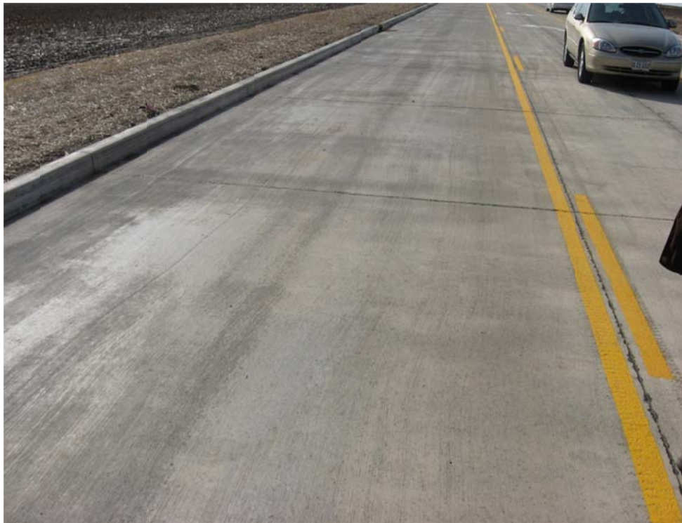
Figure 15. Eastbound Cruger Road, showing areas of poor surface friction, which are reflecting the sunlight.
