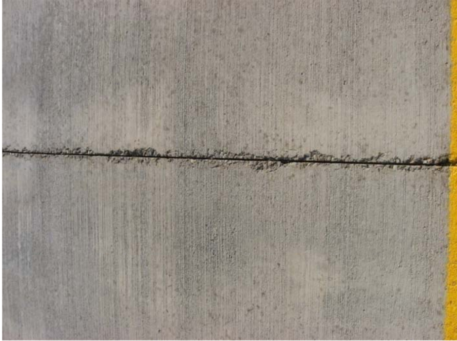
Figure 14. Excessive joint spalling on the eastbound direction of Cruger Road, as well as poor surface texture.
