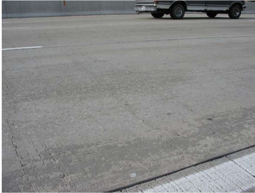
Figure 10. Closely spaced transverse cracks on Dan Ryan Expressway.
