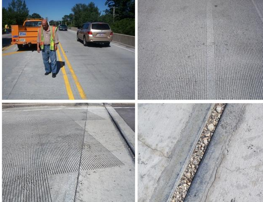
Figure 4.13. Pictures taken during the inspection of the plain and fibrous LMC overlays after 1 year in service.
