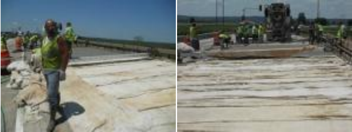
Figure 4.20. Laying down the cotton mats for curing of the fibrous FAC overlay.
