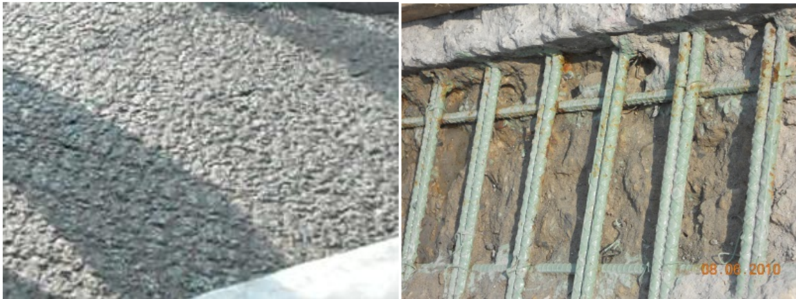
Figure 4.3. Prepared bridge deck surface using hydro-demolition (in some locations, the epoxy-coated steel bars were exposed as shown, and touch-up coating was then applied).
