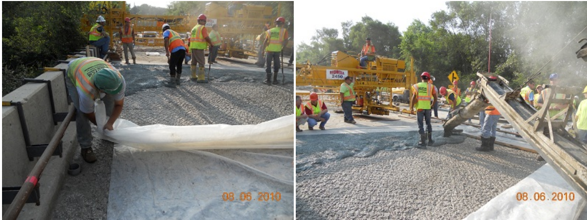
Figure 4.7. Removal of the plastic sheets that were used to keep the prepared slab surface dampened prior to installation of the overlay, starting from the transverse joints.
