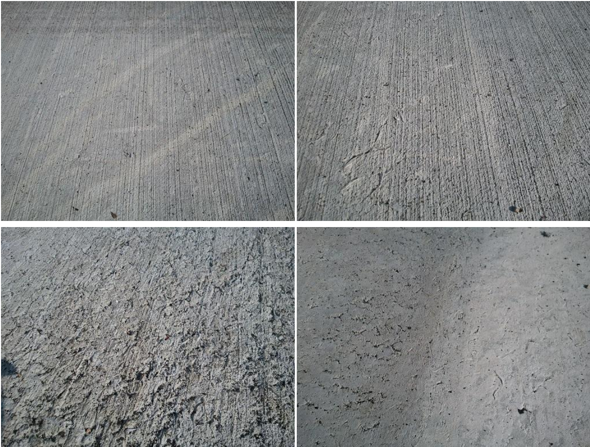
Figure 4.21. Pictures taken by the RE just before opening the fibrous FAC to traffic at the end of the curing period (1 week after the installation).
