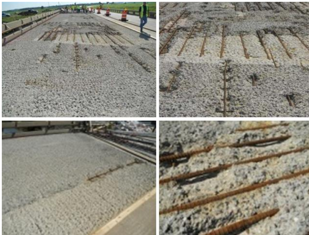
Figure 4.16. Prepared bridge deck surface using hydro-demolition (in some locations, the slab was severely deteriorated, which required exposing the steel rebar).
