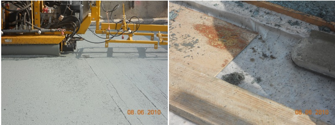
Figure 4.10. Removal of any fiber clumping during the finishing of the LMC overlay (clumping was noticed on rare occasions—probably only two times).
