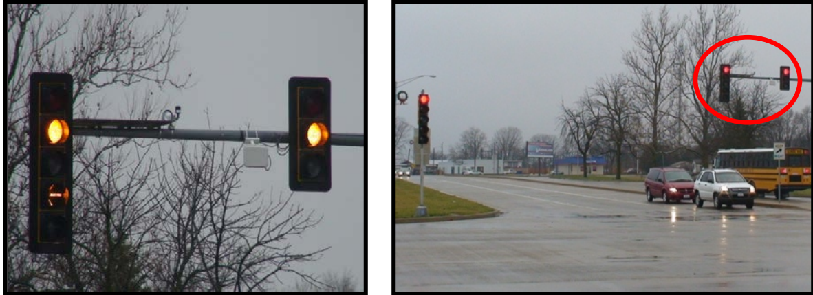
(a) Wavetronix Matrix on westbound mast arm overlooking the stop bar zones of eastbound lanes
