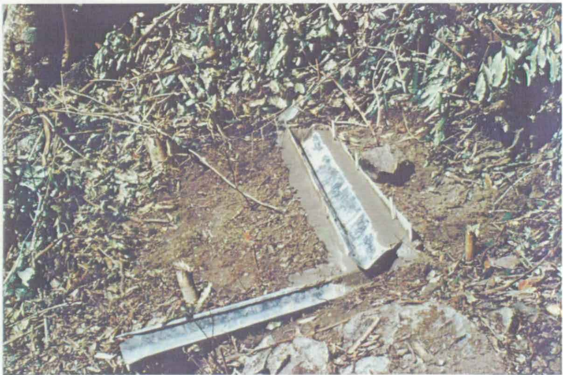
Fig.6. Erosion trough and gutter with freshly laid front lip (the metal strip is removed when the cement is set).
