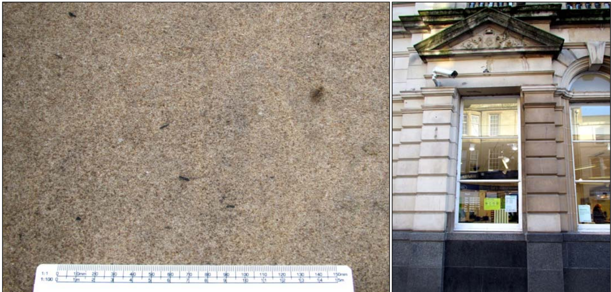
The photograph at right shows SBM5 indents to the right of the window.
