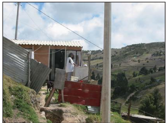
A newly installed tap after the regularisation of the water supply (August 2001).
