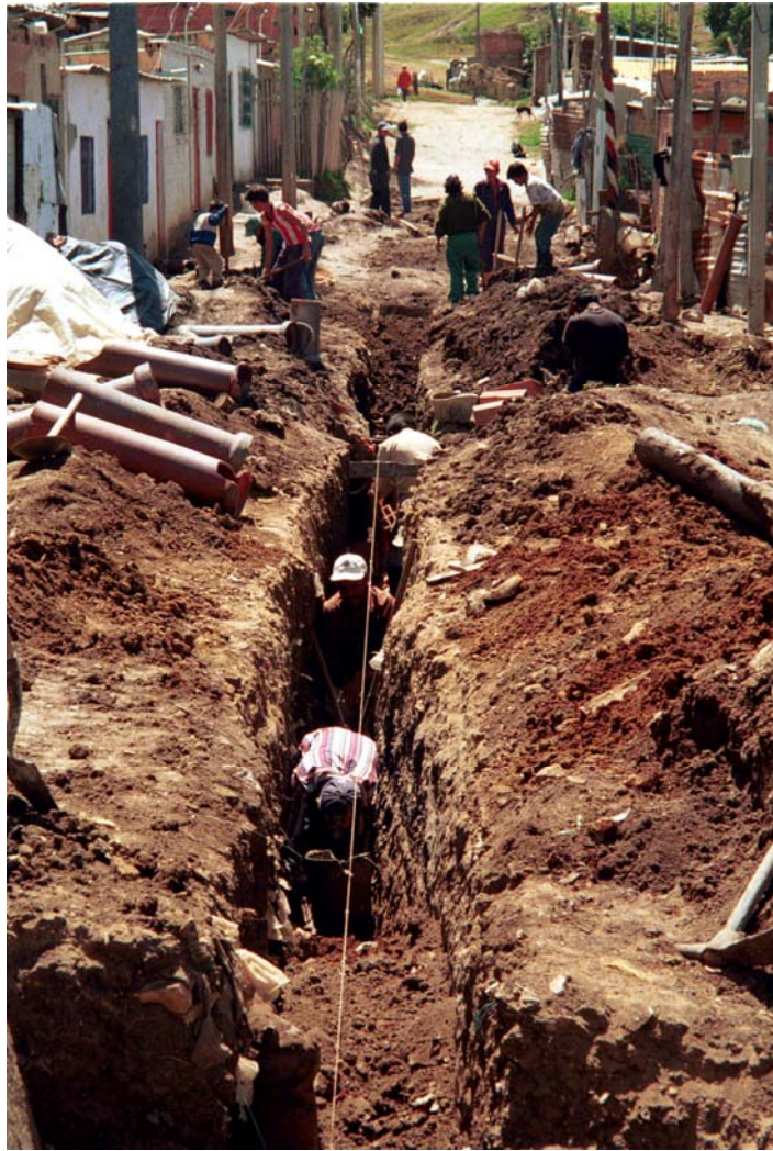
Photograph 1. Communal work to build a provisional sewerage system in Bella Flor (February 2000).
