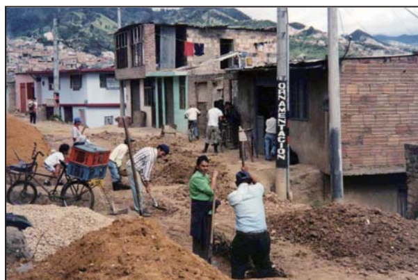
Community participation in a paving project financed by the Bogotá South Project (February 2000).
