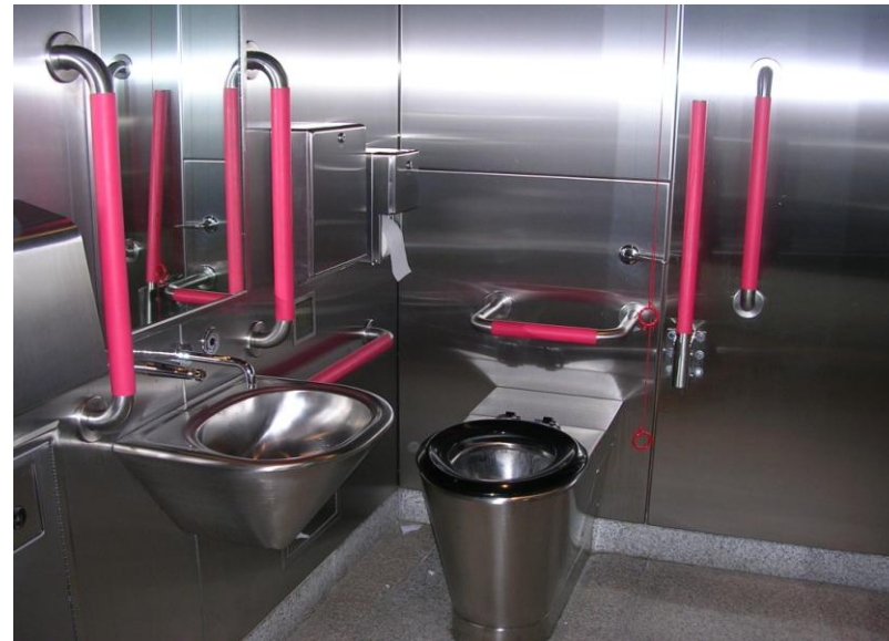
These modern toilets show a good configuration and use of grab rails. (Bichard 2004) VivaCity 2020
