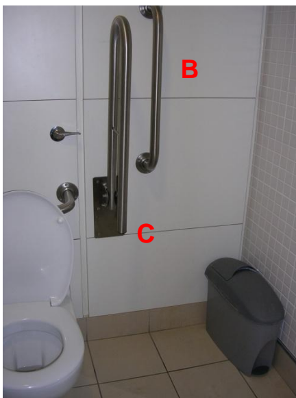
Grab rail C. Stainless steel is not the best material for this rail. (Bichard 2005) VivaCity 2020
