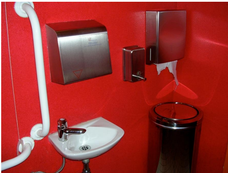
Paper towels should be provided in addition to warm air dryers. Note incorrect positioning of soap dispenser. (Bichard 2006) VivaCity 2020
