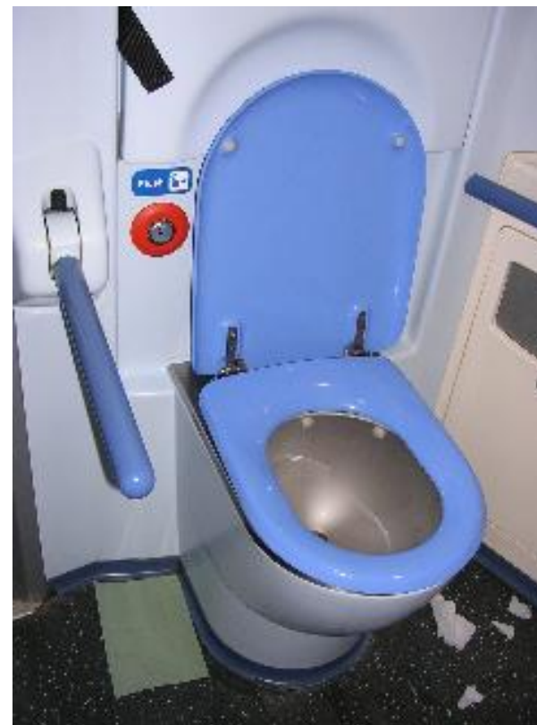
Sensor and automatic flushes can be disconcerting for users of accessible facilities. (Bichard 2004) VivaCity 2020
