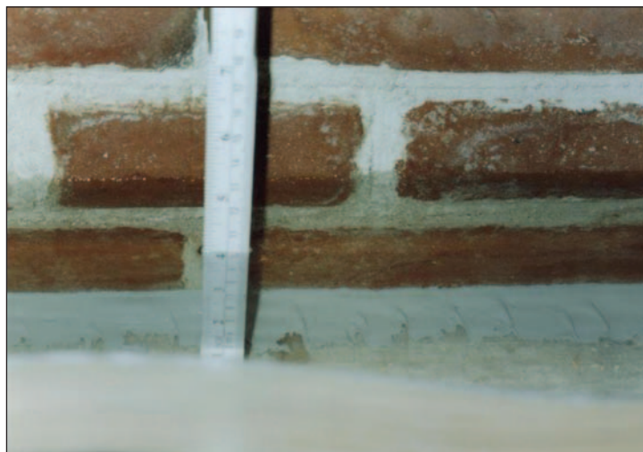
Figure 19 Flooding of brick wall
