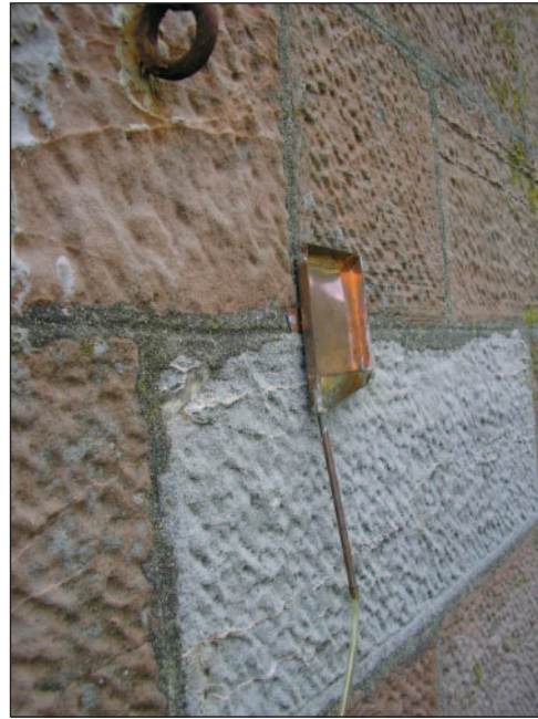
Figure 4 Driving rain collector plate mounted on east wall of Tower
