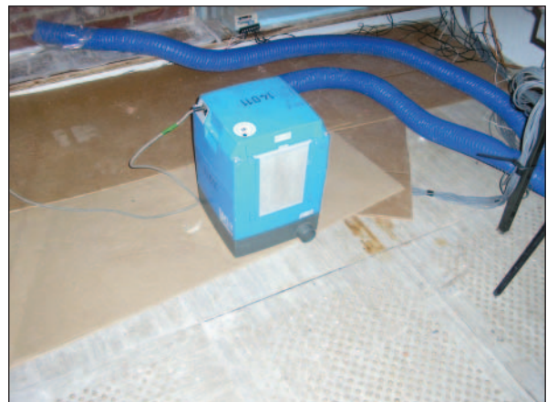
Figure 22 Dessicant wheel de-humidifier connected to enclosure by flexible hose
