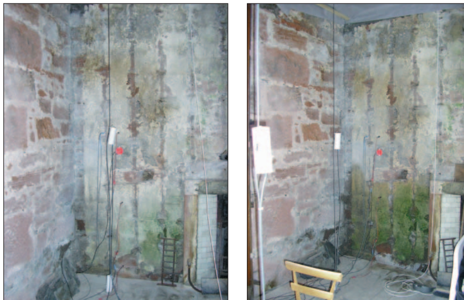
Figure 31 Spread of algae on west wall: (left) July 2004; (right) May 2006
