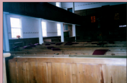
Figure 4 Flood damage to Jireh Chapel – some staining can be seen © Noel Shields
