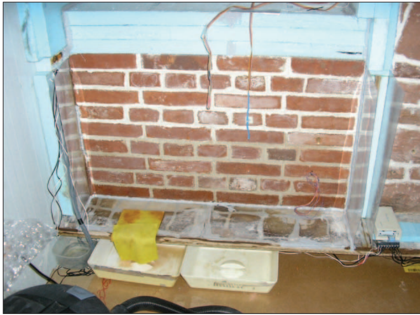
Figure 20 Warm side of brick wall showing penetration of water and evidence of damp after flooding (1 December 2005)
