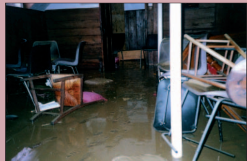
Figure 3 Flood damage to Jireh Chapel © Noel Shields
