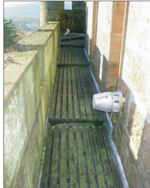
Figure 6 Photograph of the external walkway around the tower showing lead chased into stonework
