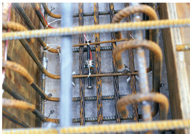
Figure 3.42 Vibrating wire gage and instrumented bars in a T-beam.
