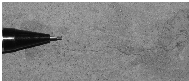
Figure 4.57 Small crack caused by expansion of Plexiglas during heating of ponding slabs. The diameter of the lead in the mechanical pencil was 0.5mm (0.02in.).
