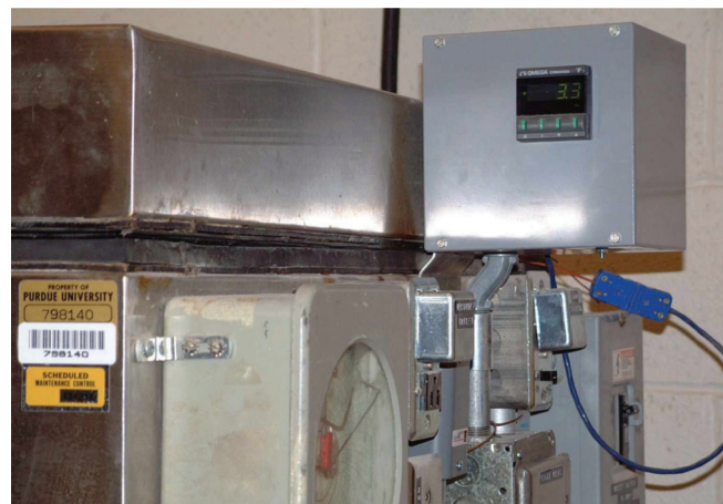
Figure 3.7 A new Omega CN9111A temperature controller installed on an existing freeze-thaw machine. The digital display on the controller is showing 3.3°C.
