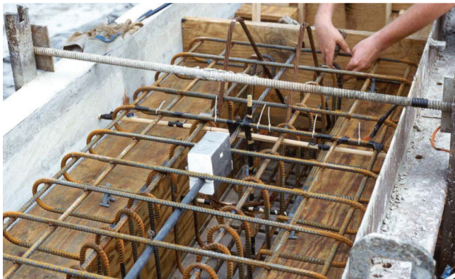
Figure 3.38 Styrofoam blockout to enable cutting of the top strand before testing and plastic de-bonding sleeve on the top strand.
