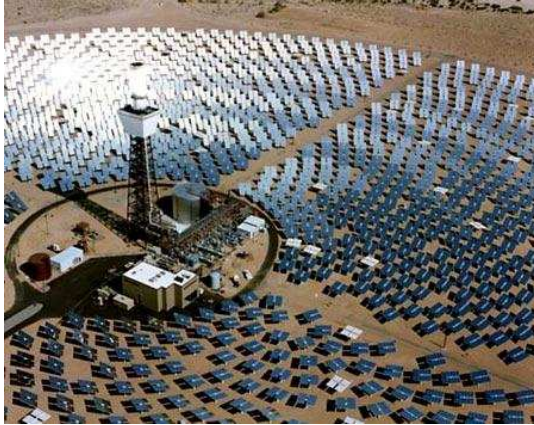
(a) Solar energy power plant
