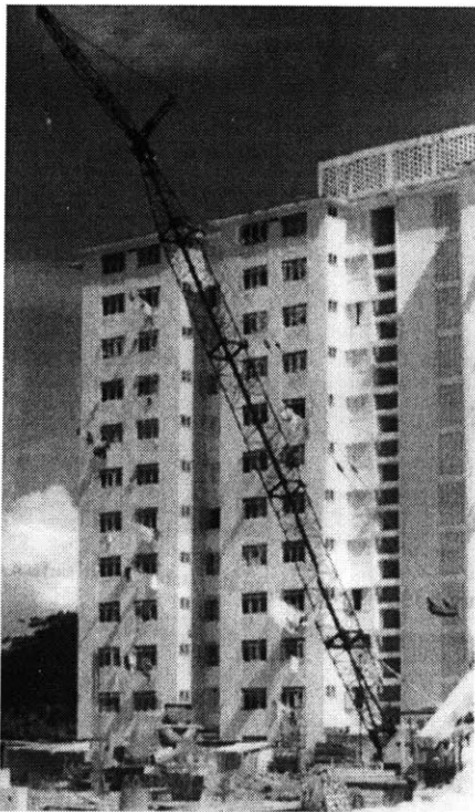
Figure 19 Typical mobile crane
