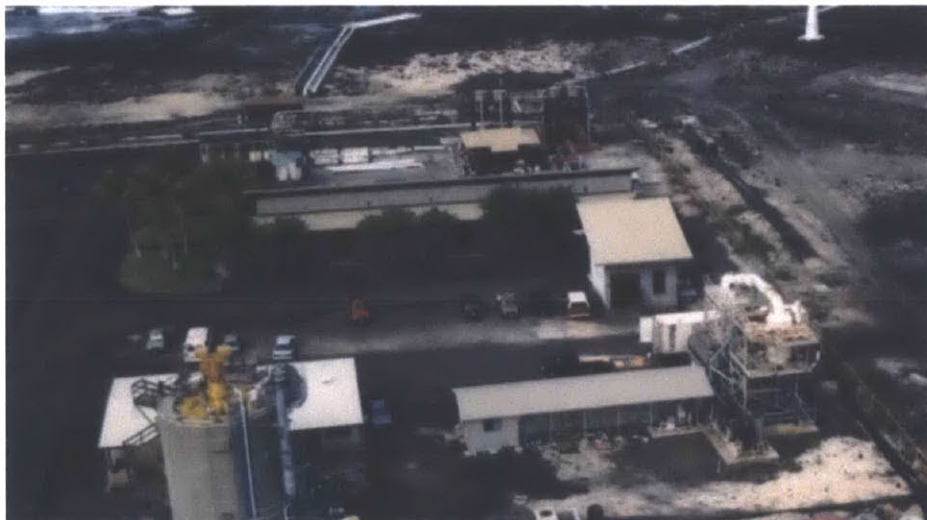
Figure 1.11 - A land based OTEC facility at Keahole Point on the Kona coast of Hawaii (United States Department of Energy).
